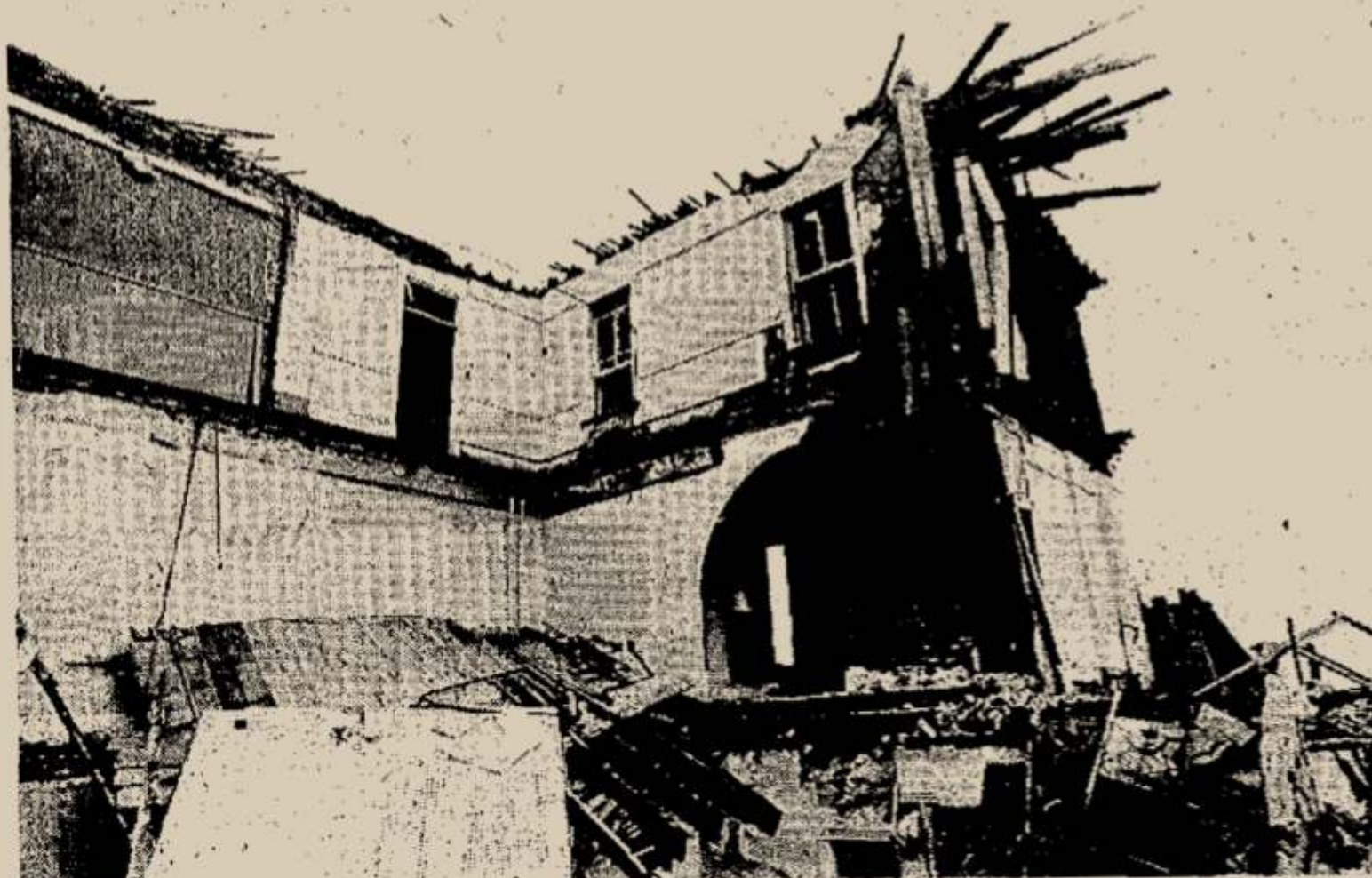
AND THE WALLS CAME TUMBLING DOWN — The Armstrong Construction Co. of Great Falls has quite a bit of work yet to do on a two-year
